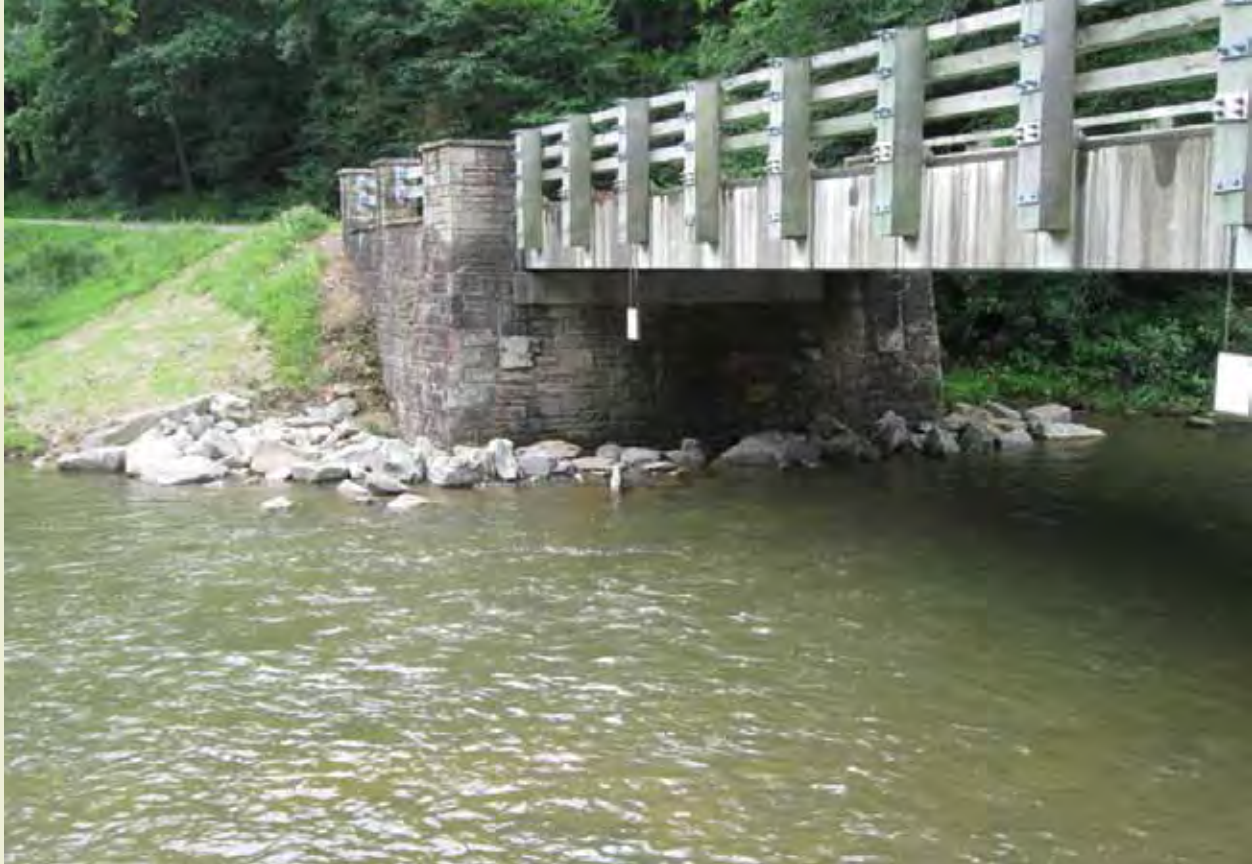
Scour protection, Laurel Hill State Park
