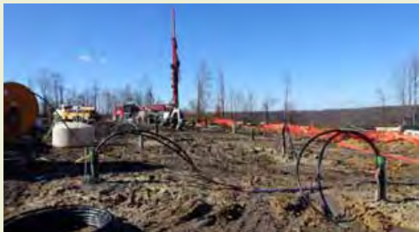
Geothermal heating system, Kinzua Bridge State Park
